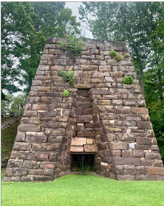
Front of the furnace
